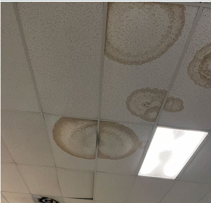
Figure 8. Stained Ceiling Tiles
