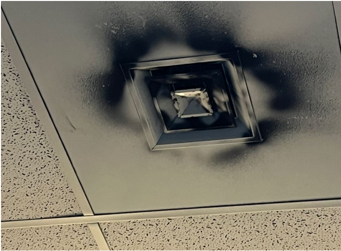
Figure 7. Black Stains on Ceiling Vents
