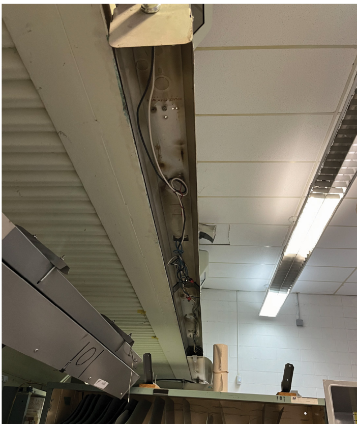
Figure 10. Several Broken Light Fixtures, with Exposed Wires, over Carrier Cases
