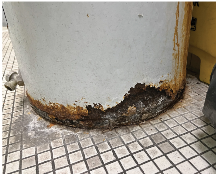
Figure 8. Non-Functioning Water Heater with Rusted Through Base
