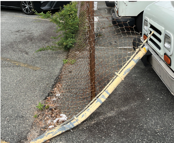
Figure 9. Bent and Damaged Metal Fence Post at the Mail Vehicle Parking Lot
