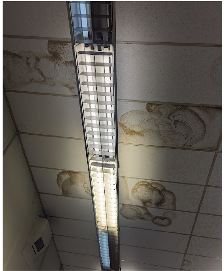
Figure 7. Water Stained and Damaged Ceiling Tiles over Workroom Areas
