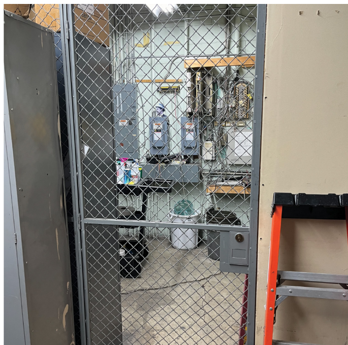
Figure 5. Electrical Panels Inaccessible and Locked in Security Cage
