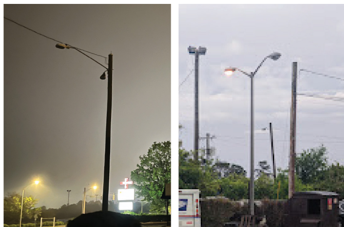
Figure 6. Lights Over Customers and Employees Parking Areas Were Not Lit
