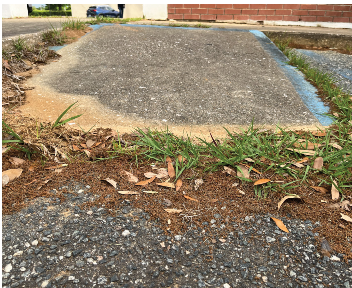
Figure 4. Handicap Accessible Parking Ramp with Tripping Hazard
